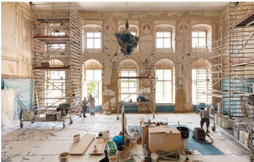
In the course of a comprehensive renovation project, construction defects from previous decades were addressed, period wall paintings uncovered and sealed asphalt pathways removed from the courtyard.
