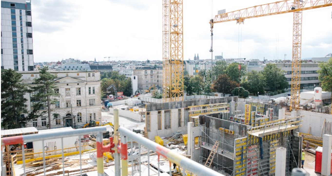
The major new construction projects at MedUni Vienna were in full swing in 2023.
