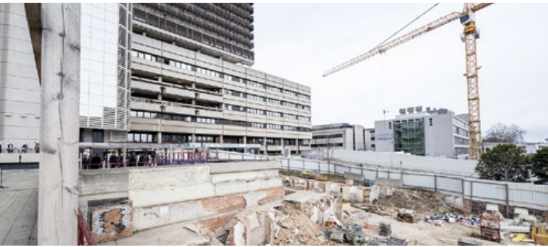
The foundation pit for the Center for Translational Medicine was completed and the base plate laid in mid-October 2023.
